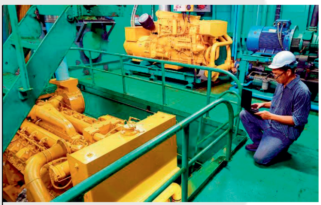
Marine: Having accurate real time data is essential for self-sufficient maintenance on vessel.
